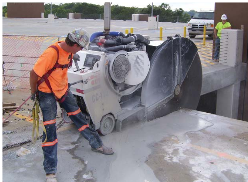
The contractor was 110 feet above ground level while cutting the fourth story of the structure.
