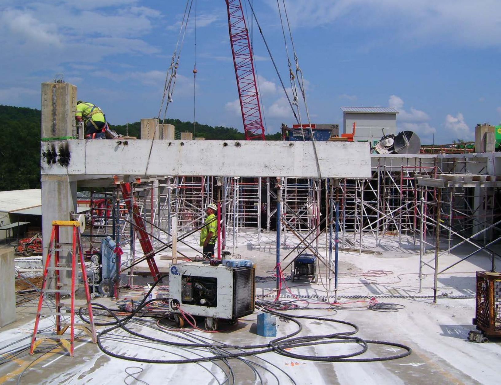
Slab decks, beams and piers were removed so that the existing parking garage could link to a new hotel and casino building.
